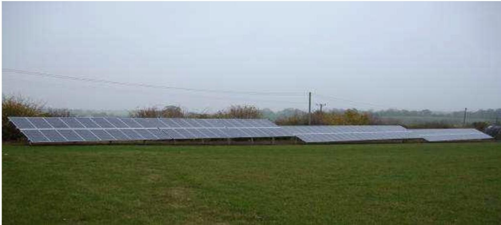
Photo of an installed 30kW ground mounted PV system.
